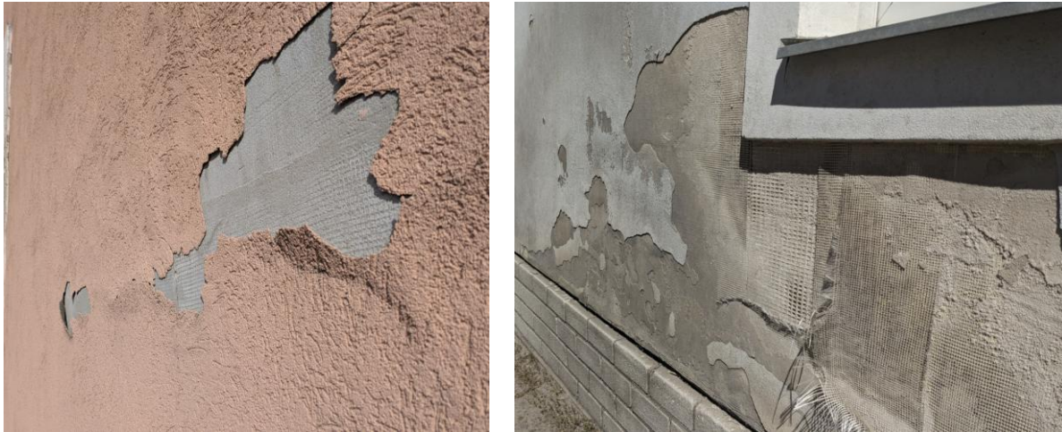
Figure 6: Examples of damage in ETICS facades: loss of adhesion between finishing and reinforcement layers (left) and extensive frost damage (right). Photos: Paul Klõšeiko.
