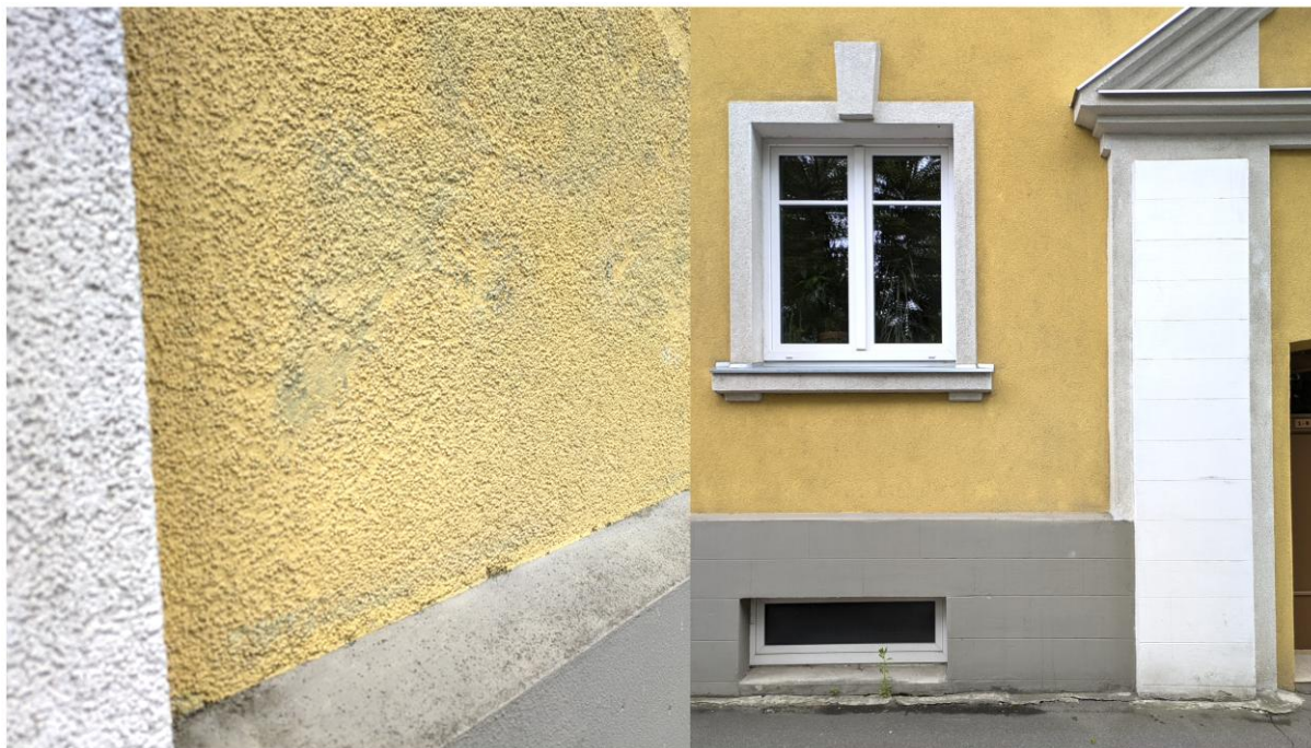
Figure 4: Finishing plaster with uncharacteristically large grain size can ruin the final result of the exterior insulation works (photos: Paul Klőšeiko).
